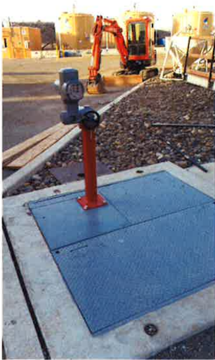
Photo 1-1 Electric Actuator Installed on Existing Vault
